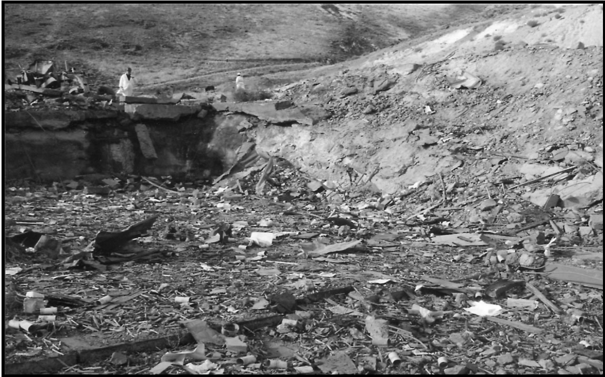
Figure 7. Booster Room 2 After Explosion
