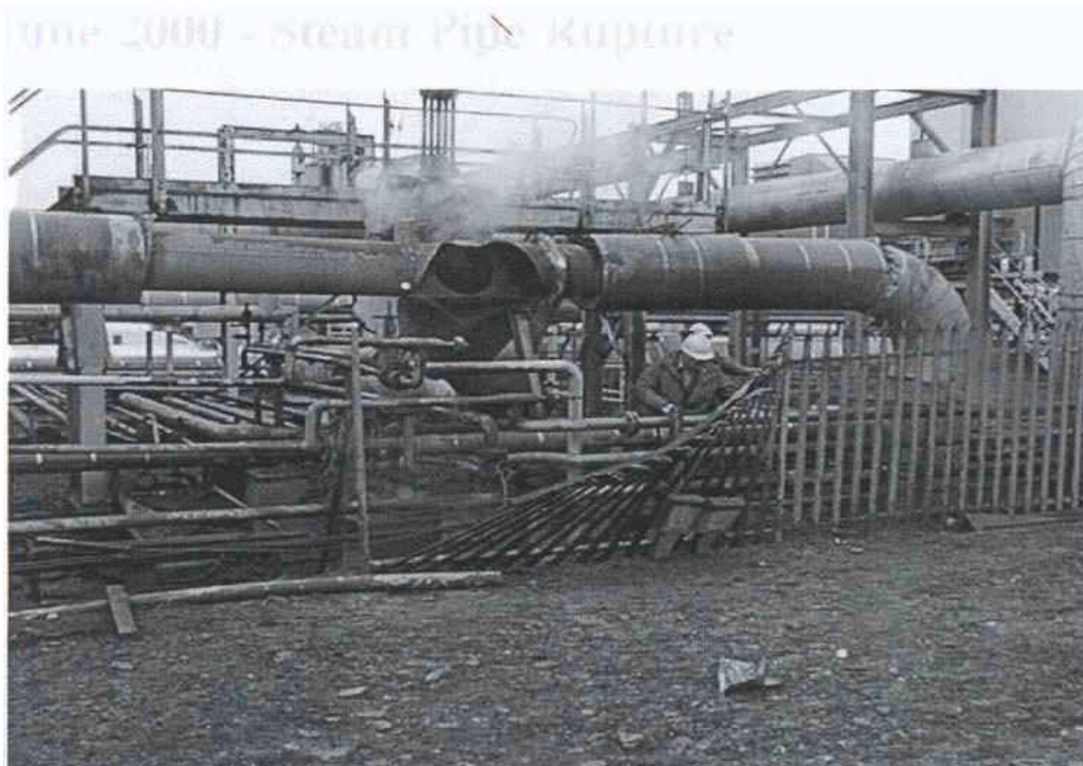
Figure 12 – Steam Main Photo
