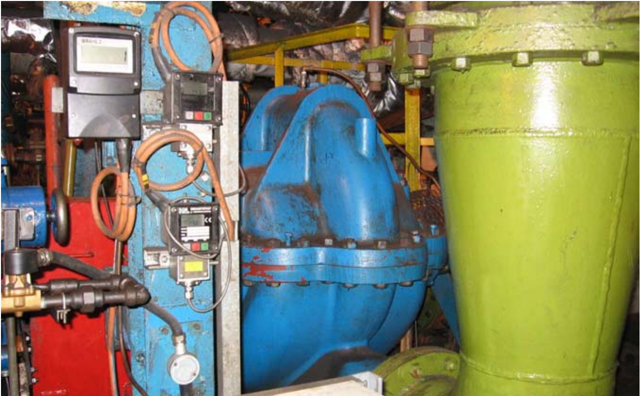
Figure 7 Furnace steam turbo water pump
