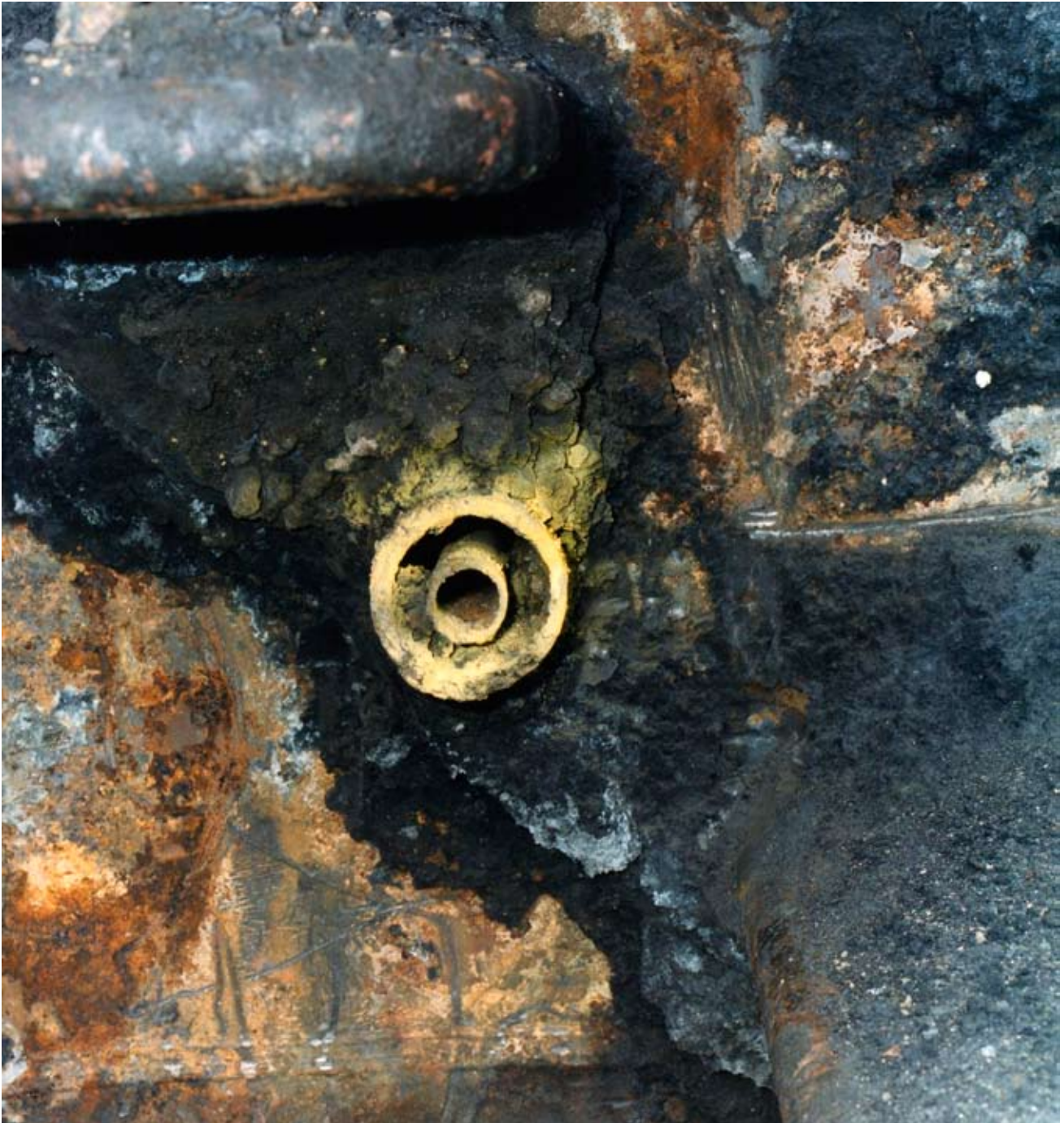
Figure 12 Example of burnt-out Sorrelor cooler
