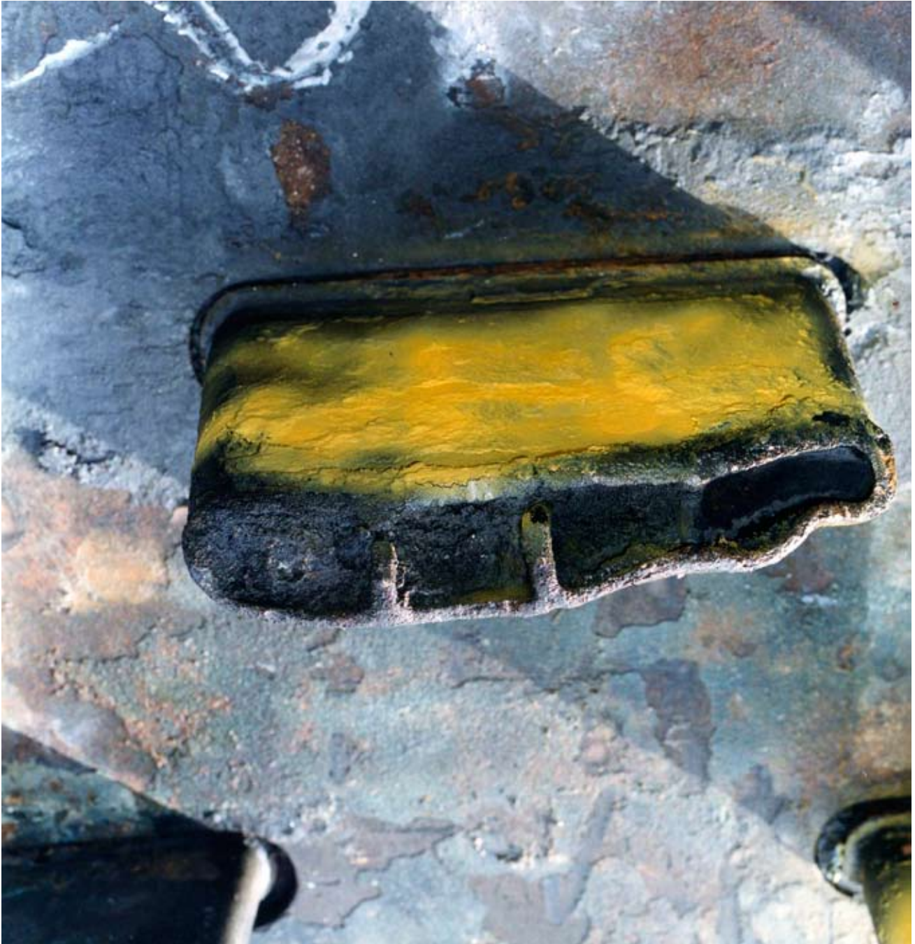
Figure 13 Example of burnt-out plate cooler
