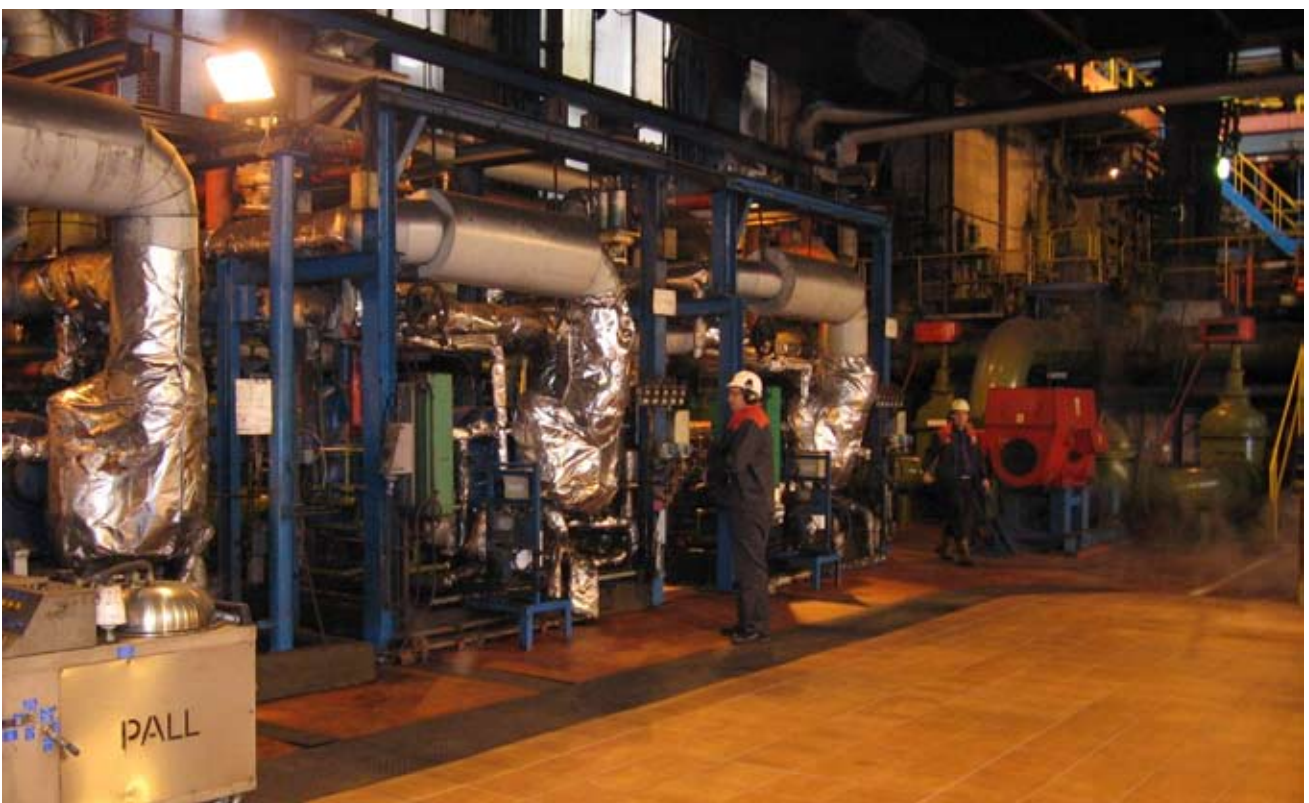
Figure 6 Margam B Power Plant showing furnace water pumps
