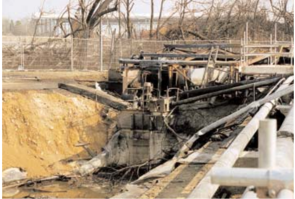
Figure 11 The three parallel bars show where the pumphouse stood before the incident
