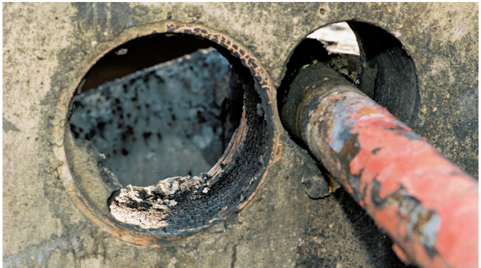
Figure 9 Loss of sealant between penetrating pipe and bund wall
