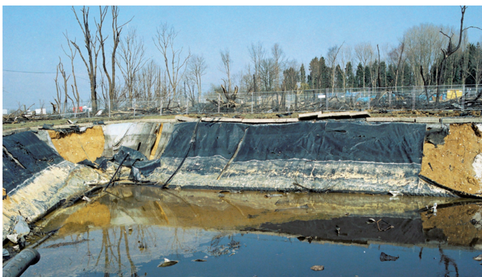
Figure 11 The firewater lagoon on the HOSL site after the incident
