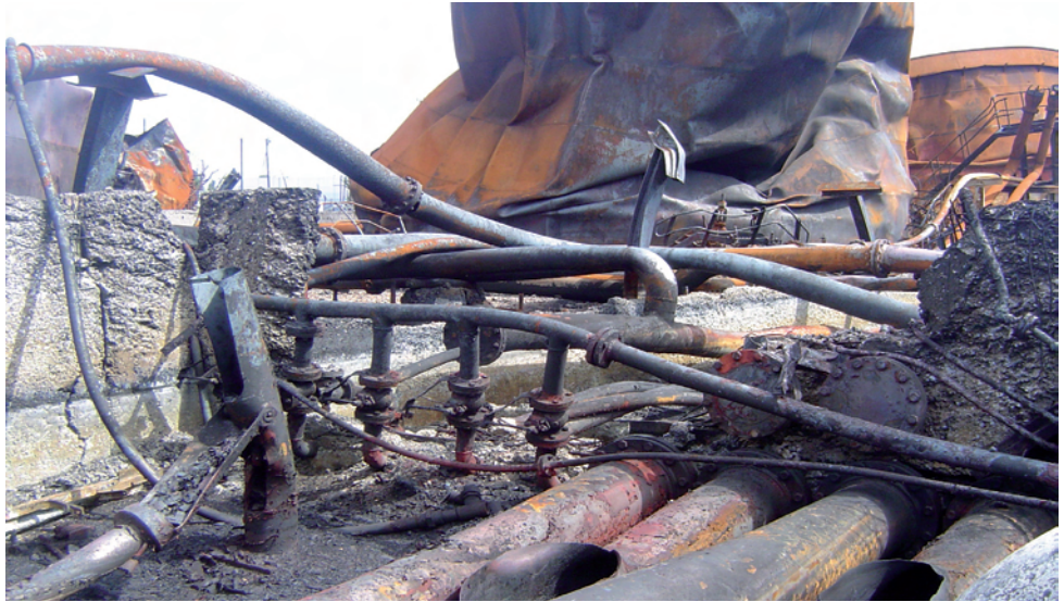
Figure 8 Catastrophic bund wall failure at pipe penetrations
