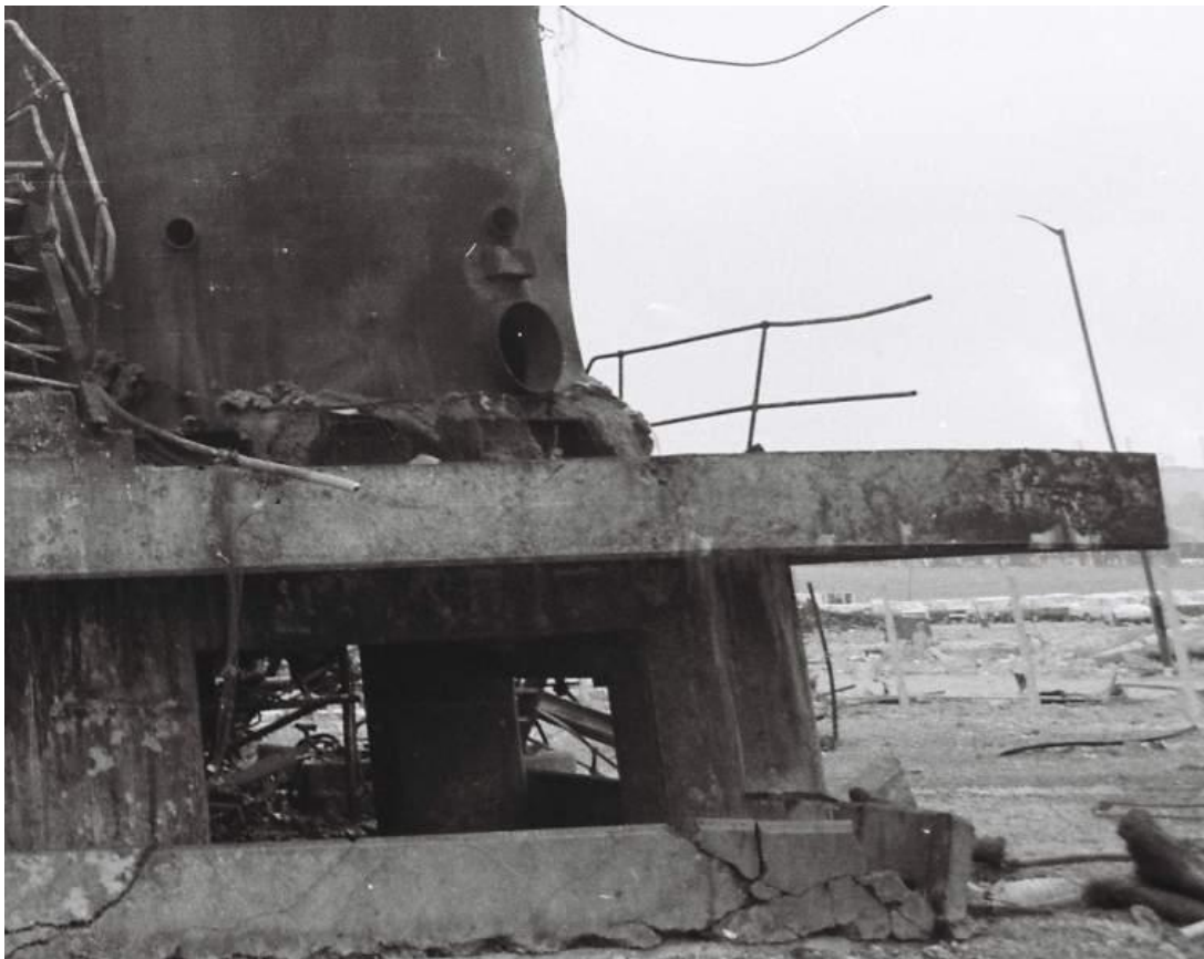
Figure 12: Reactor 6 (Number 5 missing). Significant pressure damage to the skirt
