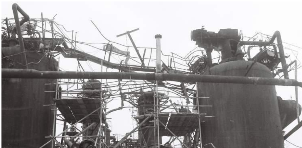
Figure 9: Openings left after loss of bypass pipe.
