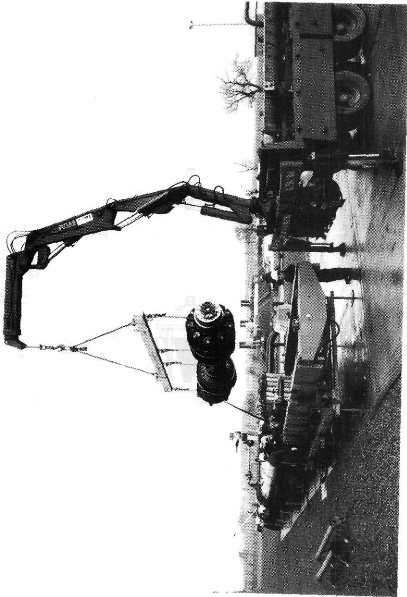
Launch / receive equipment
