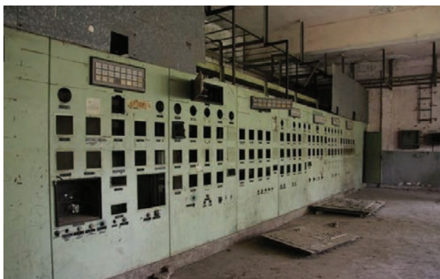
Control Room Feb 2014 (Credit BMA)
