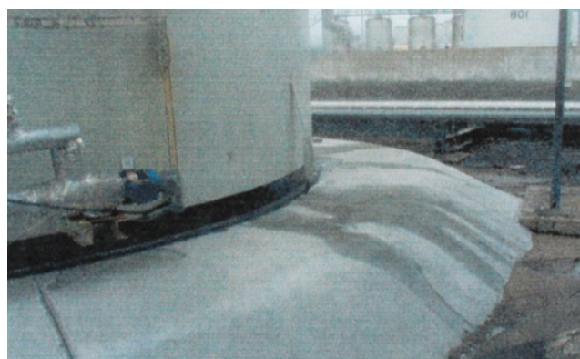
Tees storage leak: sodium cyanide leaking onto tank 713 berm – 21 July 1999.
