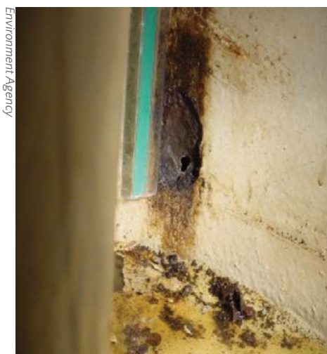
Tank 115 base internal sump and pipes (below) with erosion and corrosion causing hole in the sump wall (left)
