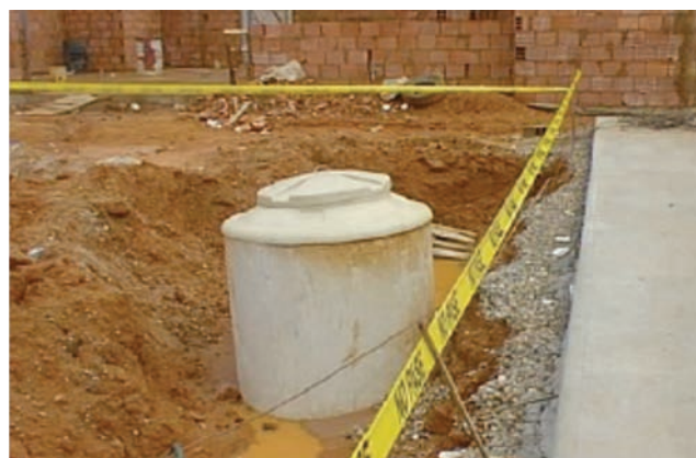
Figure 3: Underground tank with entry forbidden
