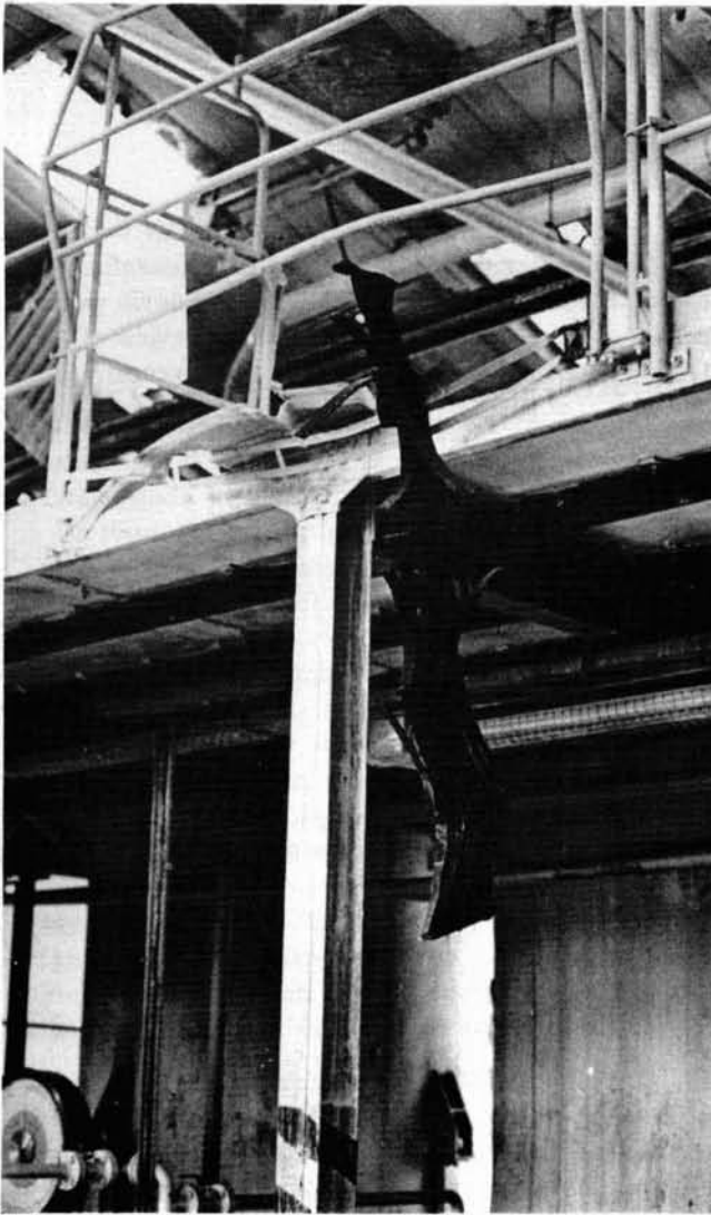
Interior of a room off the No 2 warehouse showing roof damage and a collapsed cable tray.
