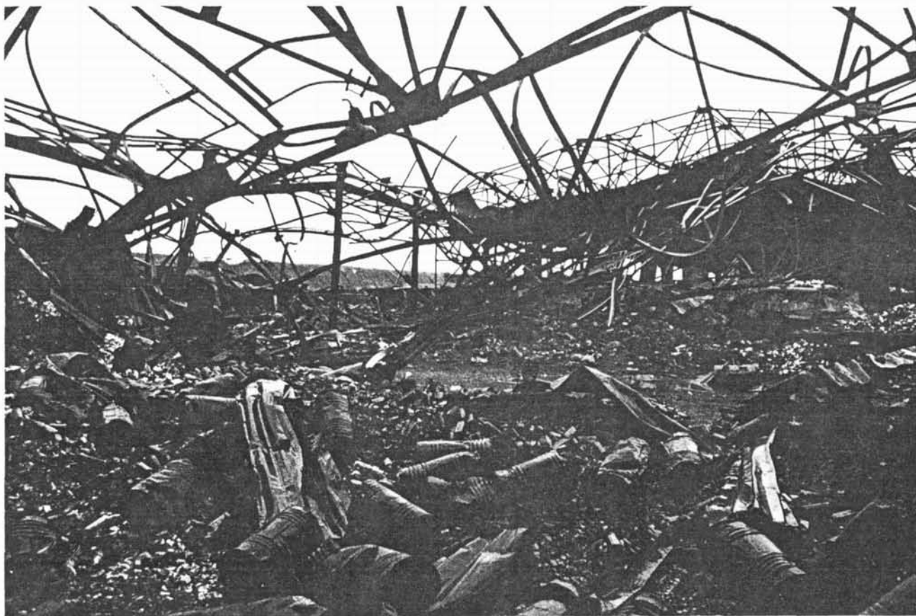
Fig 8 General view of the seat of the explosion with damaged drums of sodium chlorate in the foreground.
