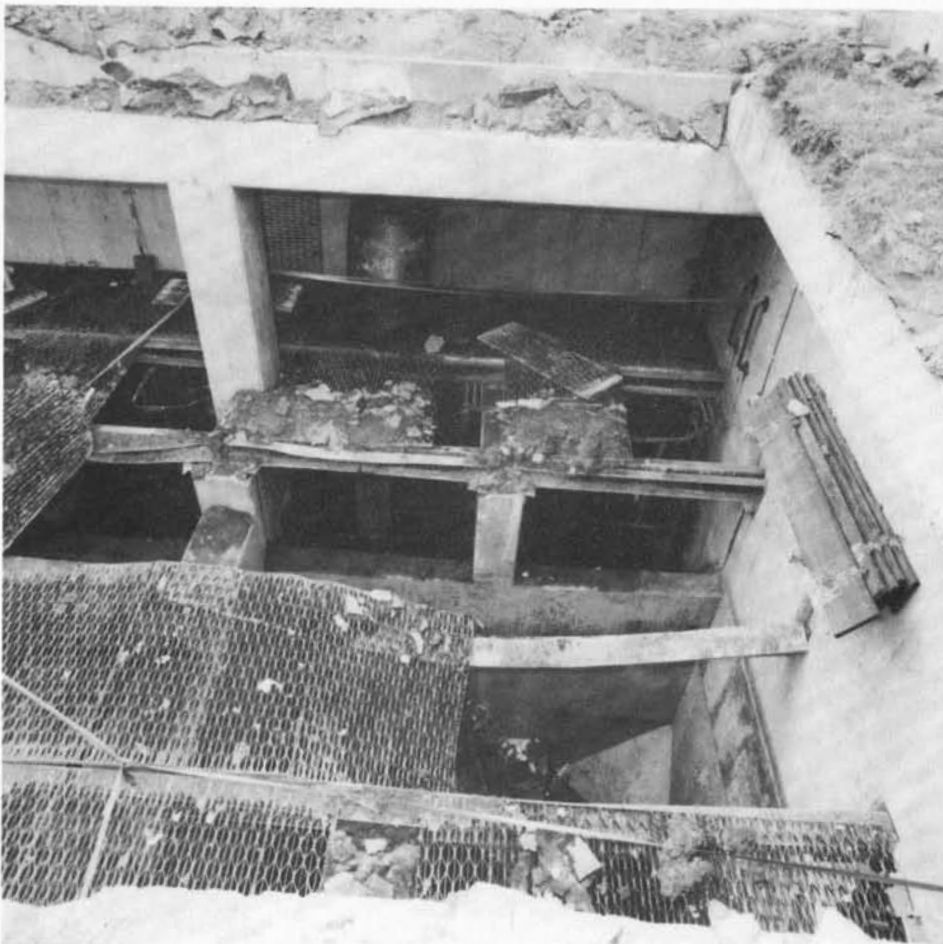
View looking towards the north-west corner of Abbeystead Valve House after removal of damaged roof beams
