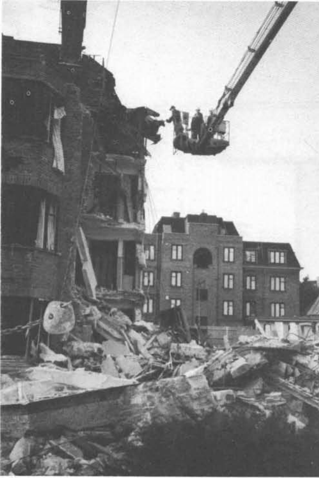
Fig 8 Mobile access platform
