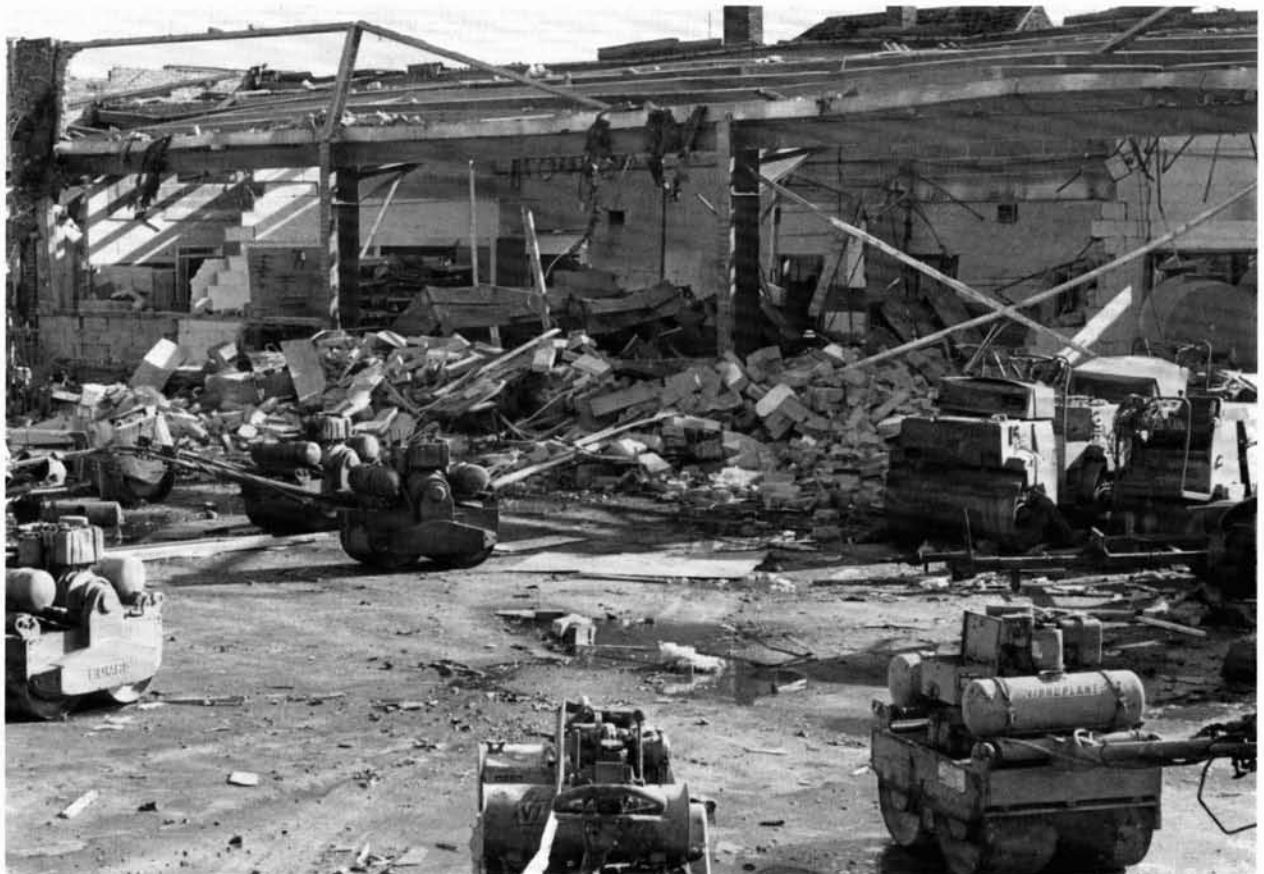
Figure 9 Blast damage to the Vibroplant building ( Photograph reproduced by kind permission of Peterborough Evening Telegraph )
