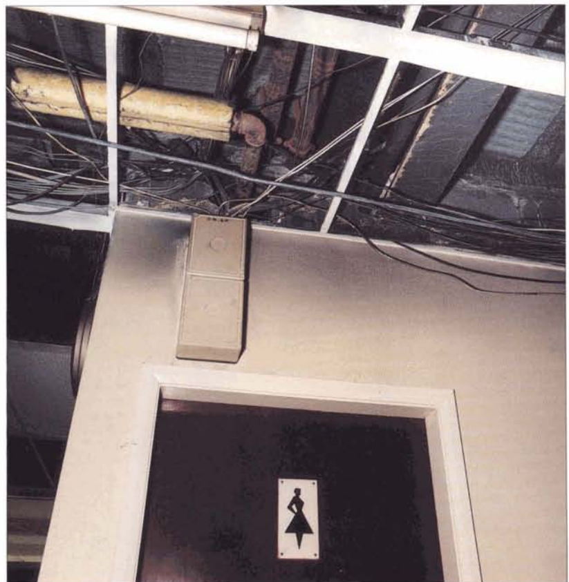
Figure 12 Photograph showing breaches in the fire-resisting enclosure around pipework and cables
