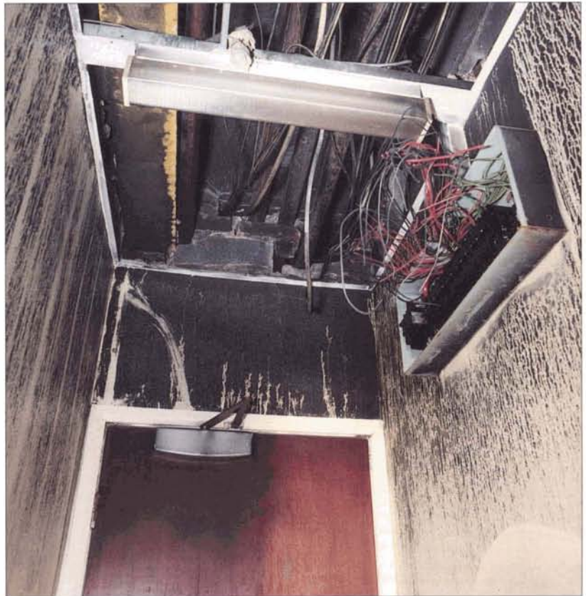
Figure 11 Photograph of smoke damage in the second floor women's toilets
