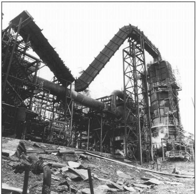
Figure 7 Some very large structures, such as the ducting weighing several tonnes shown here, were left balanced in dangerous positions after the explosion
