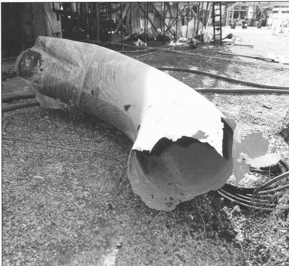
Figure 5 The 30 inch flare line elbow bend that failed and fell to the ground, releasing the hydrocarbon liquid and vapour
