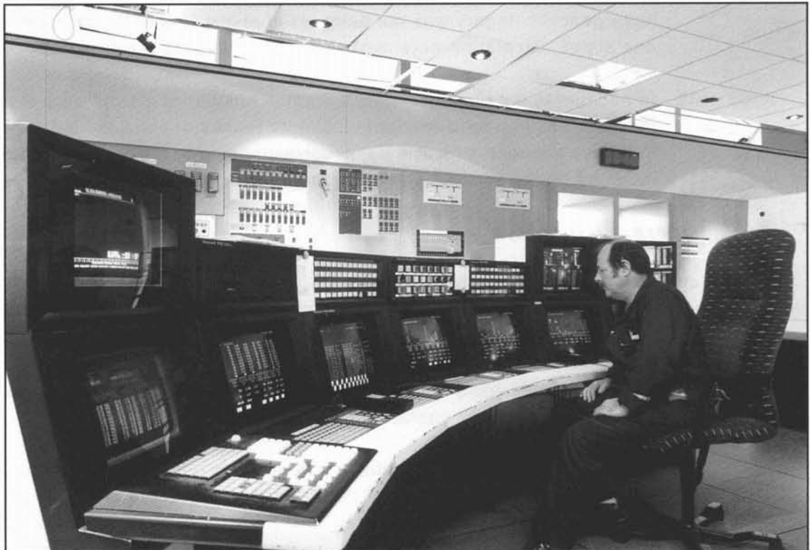
Figure 3 Part of the main control room, showing the display screens and keyboards used to operate the plant
