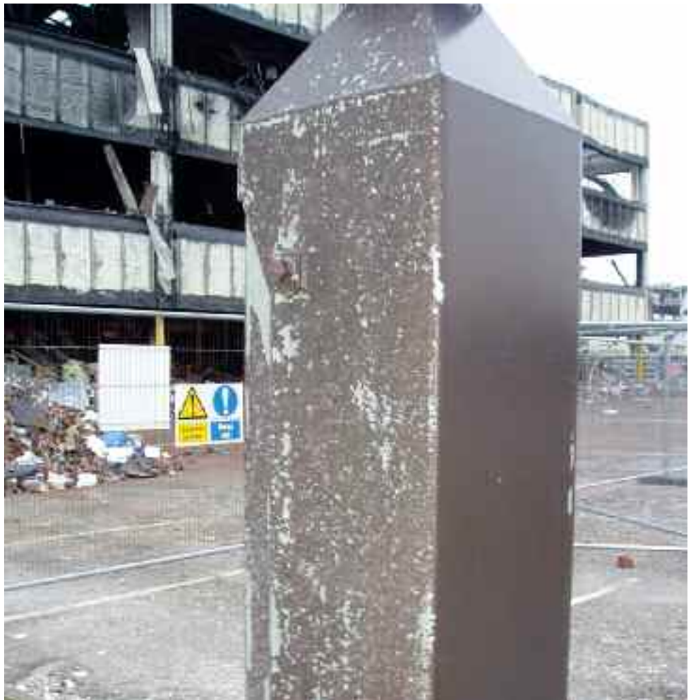
Figure 15 Steel post in the west car park of the Northgate building. The post shows abrasion marks on its south face
