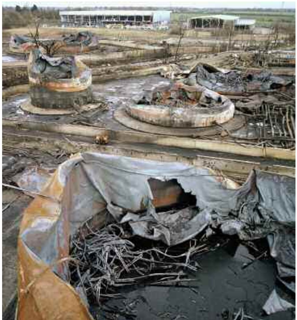
Figure 7 Looking east across the top of Tank 912. Tank 12 is in the background, across Cherry Tree Lane
