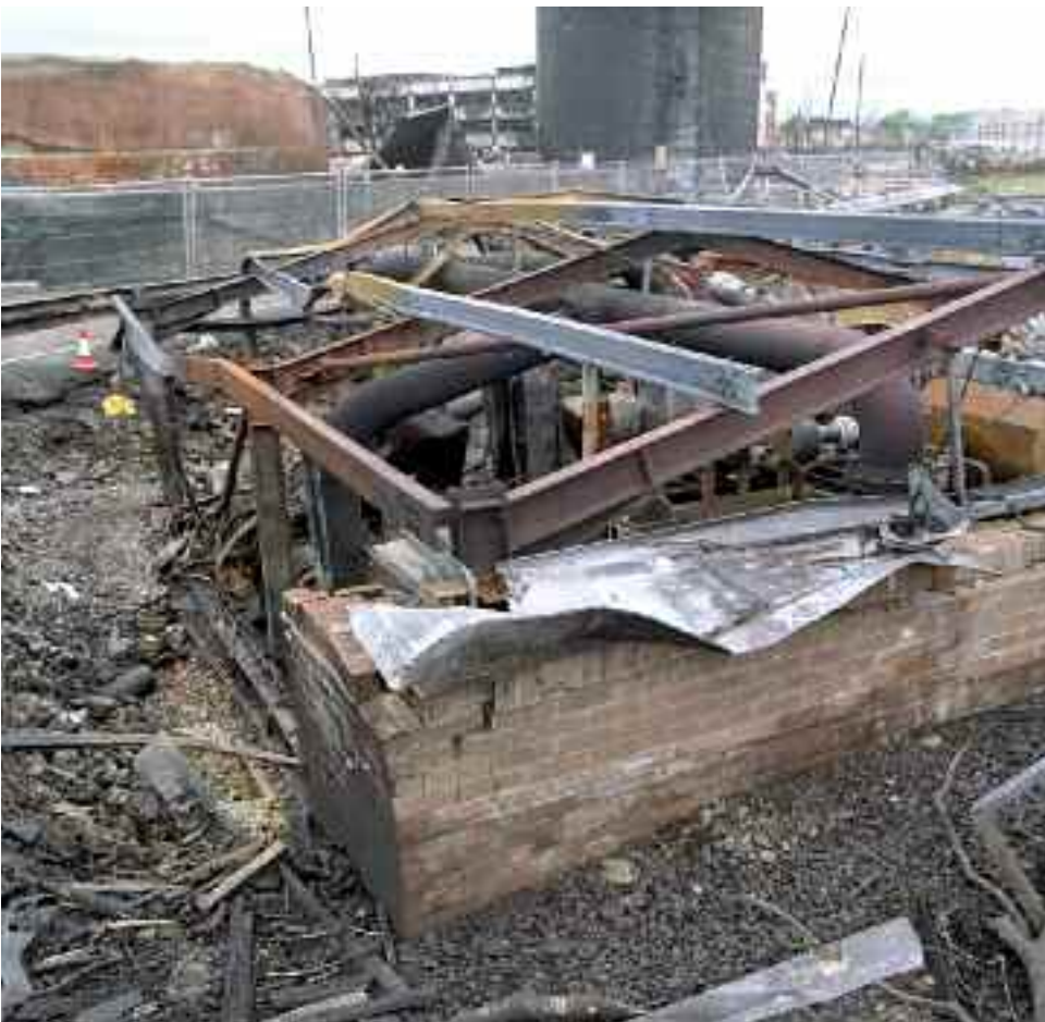
Figure 13 Emergency pump house on the HOSL West site, from its north-east corner
