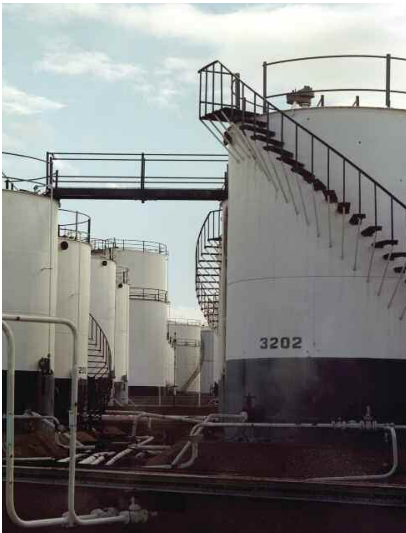
Figure 5 General view of fuel storage tanks with associated pipework and instrumentation
