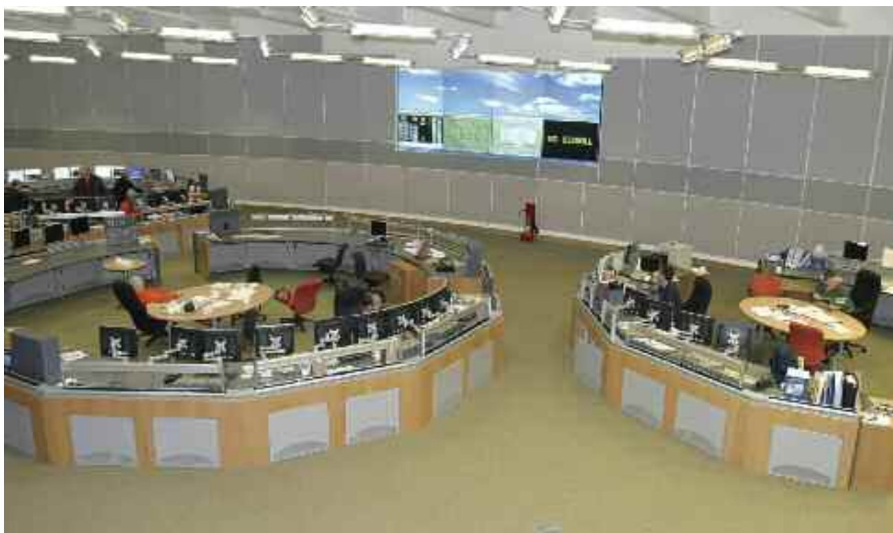
Figure 9 A modern process control room
