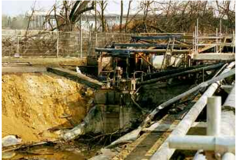
Figure 11 The three parallel bars show where the pumphouse stood before the incident
