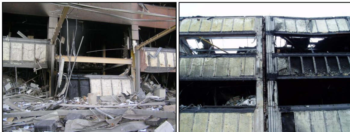
Figure 2. Photographs of blast damage to Northgate building showing detached cladding panel and flexural failure.
