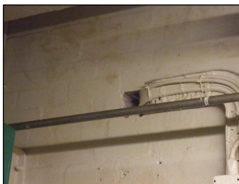
Figure 6 – Unsealed Penetration in a Fire Compartment
