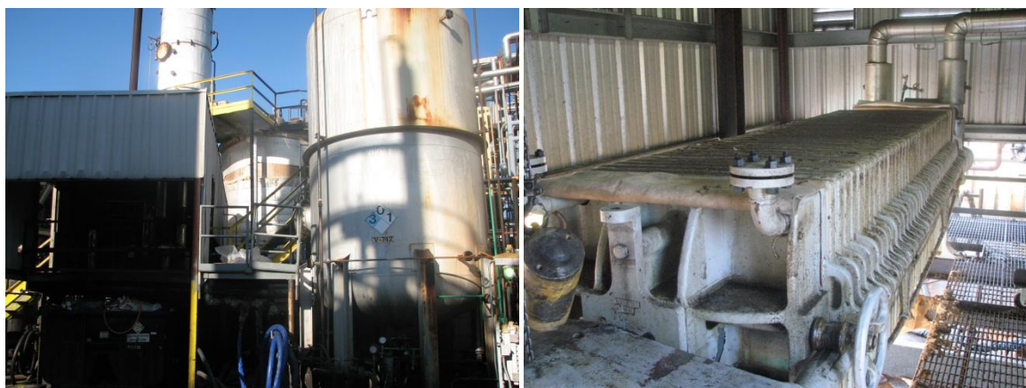
Figure 2. (left) Filter press building, adjacent bulk supply tank, and roll-off box for waste. (right) Close-up of similar filter press.
