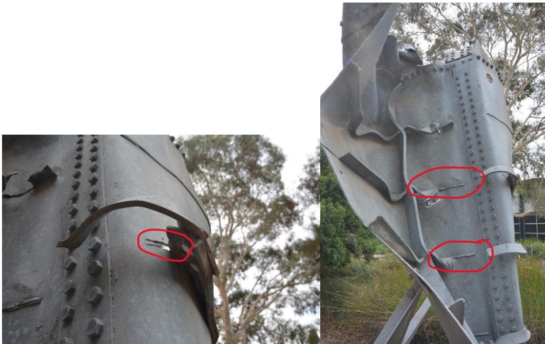
Figure 6. Section of the inner web of the box girder, shows where the steel was torn, mainly in the heat affected zones around welds.
