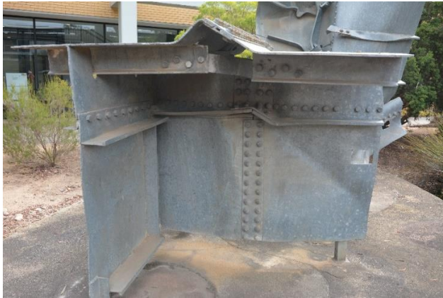
Figure 4. Shows a similar buckle that developed after the kentledges were loaded
