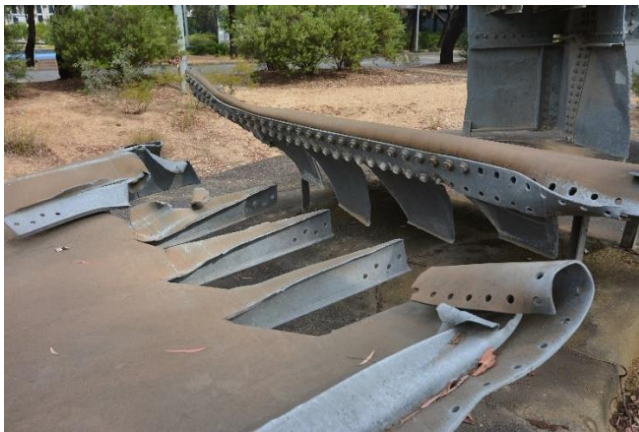
Figure 5. Shows the failure point on the flange where they had started to remove some bolts to release the stress causing the buckling. This was the failure point on the span that collapsed.
