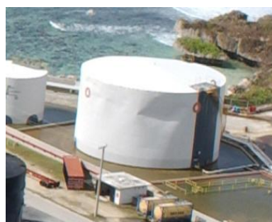
Figure 4. Shell buckling of a tank during a wind load caused by Hurricane Katrina.
