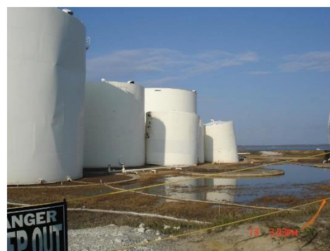
Figure 2. Shell Buckling of a tank during a flood caused by Hurricane Katrina.
