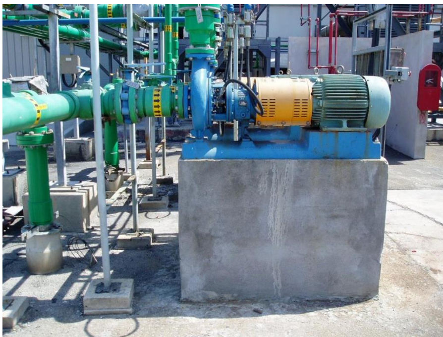
Figure 3: Example of a key monomer pump elevated above the 500-yr flood elevation.
