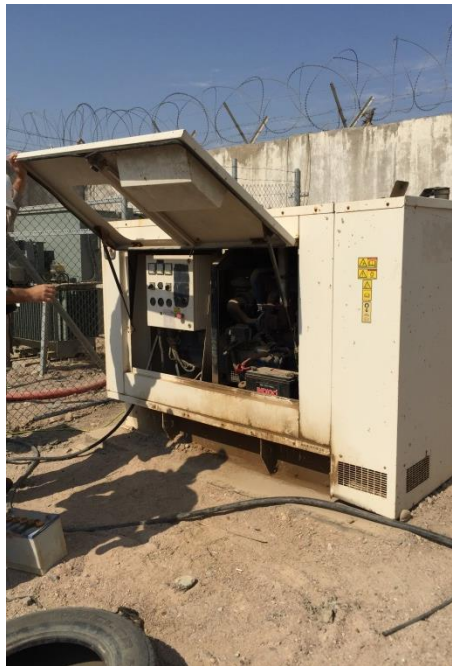
Figure 6: Diesel generator in poor condition.
