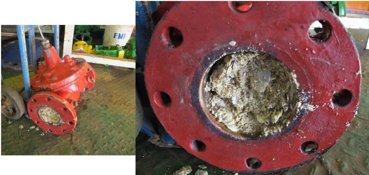
Figure 9: Fully Clogged Deluge Valve (mainly by sea shells)
