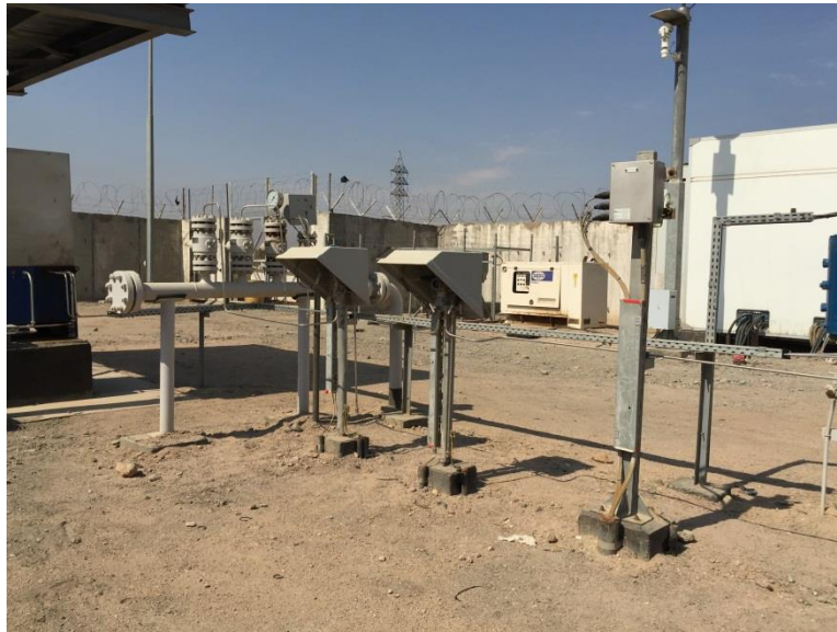
Figure 5: Proximity of temporary power supply diesel generator with pipeline topside valves and instrumentation
