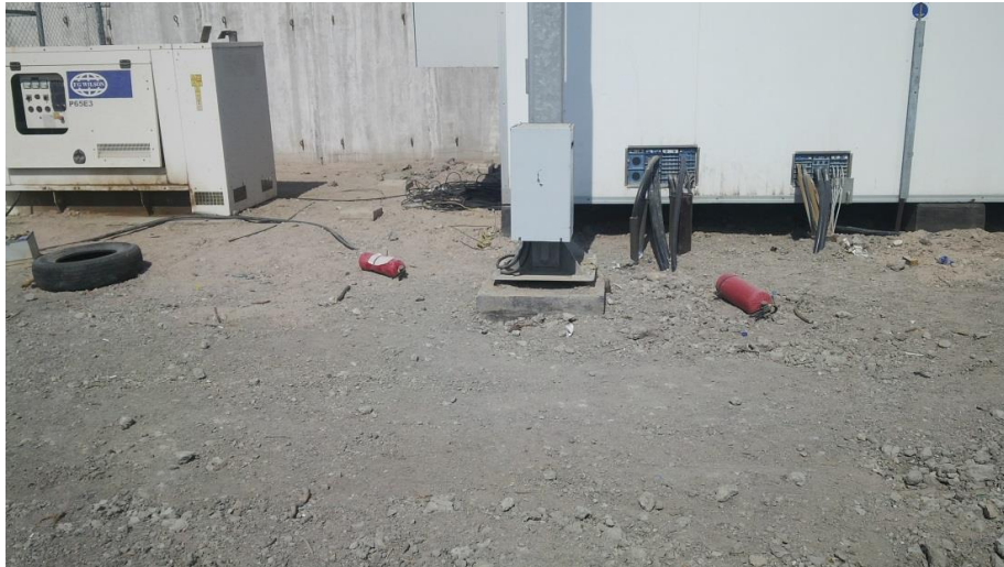
Figure 7: Damaged fire extinguishers /poor housekeeping.
