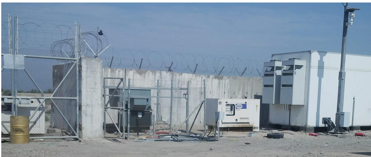
Figure 4: Current location of temporary power supply diesel generator.
