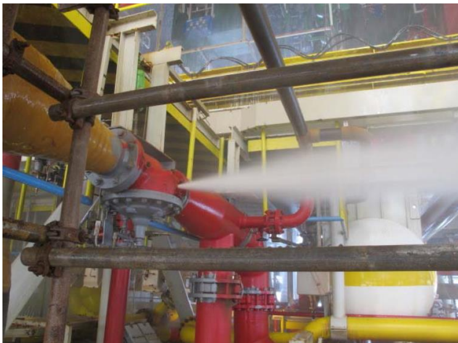
Figure 8: Water jet cause by blown plug on Deluge Valve during a Firewater test.
