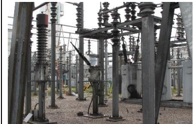
Figure 12: Ceramic metering transformer explosion, brittle failure - 250 projectiles, 0.05kg - 1.5kg, 10m to 70m
