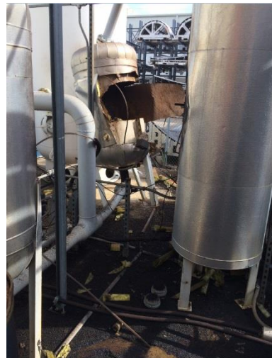
Figure 10: Failure of air purification vessel near operating pressure - no primary fragments some secondary projectiles
