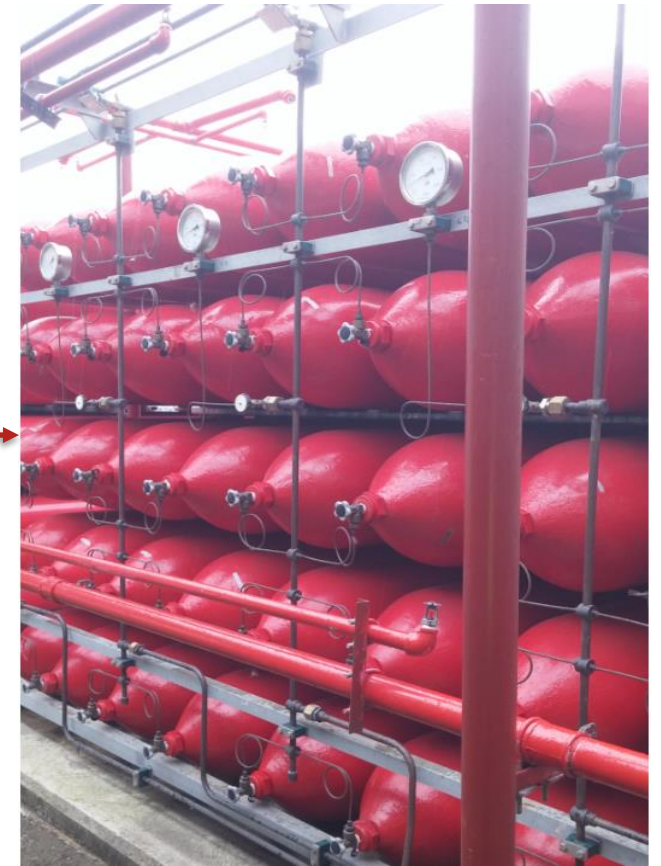
Example of hydrogen cylinders bank
