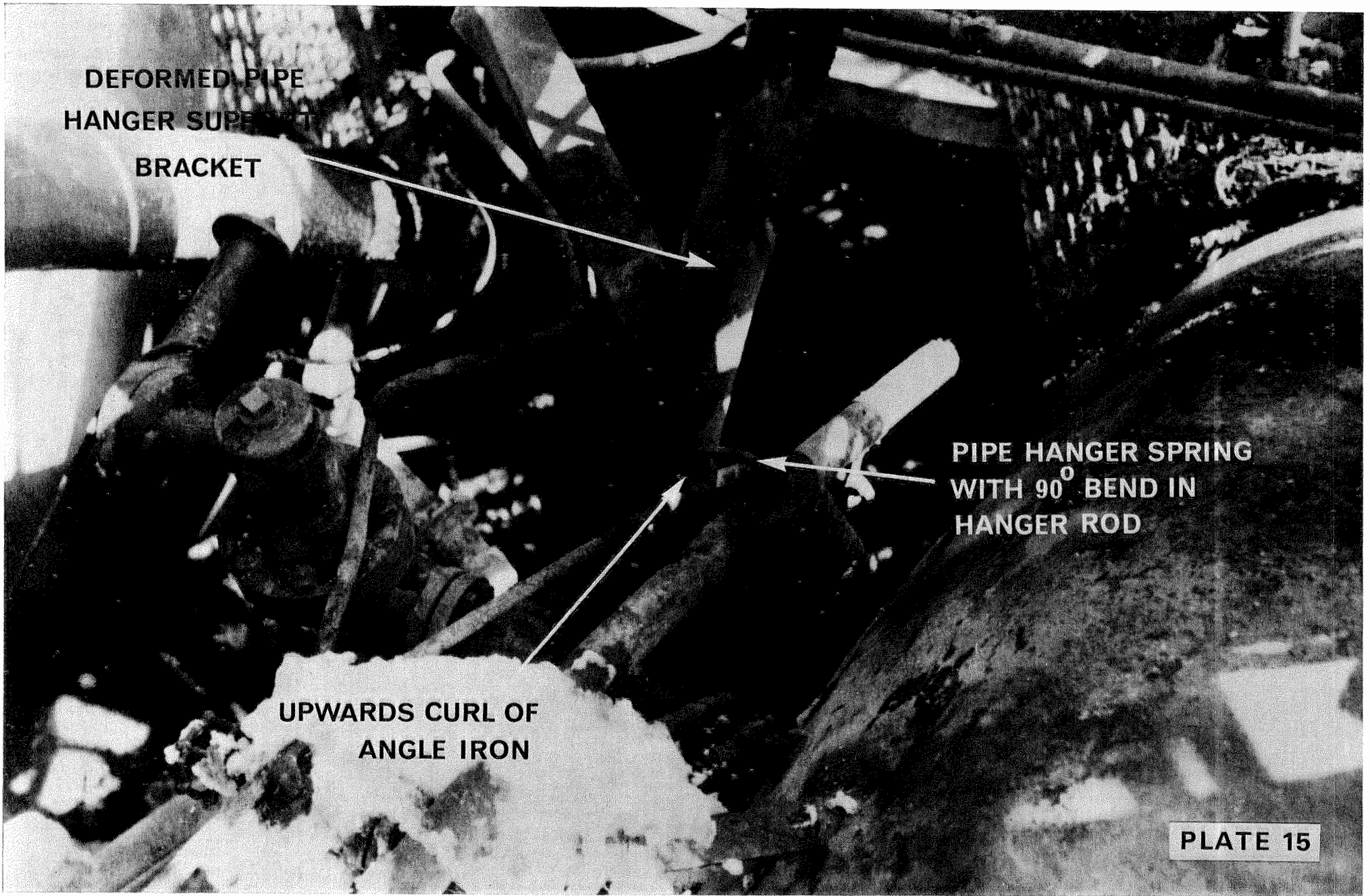
Plate 15 Broken and bent pipe hanger rod, and spring.
