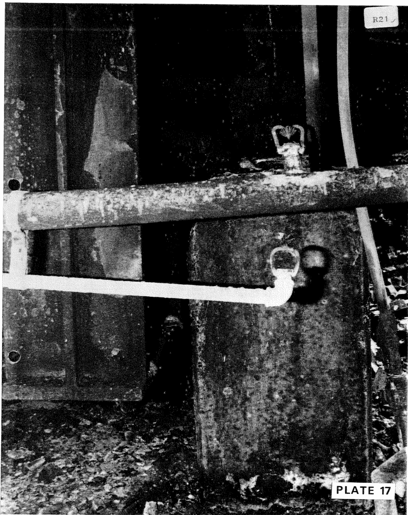
Plate 17 Typical water spray nozzle with air-operated sensor below. Photograph taken after the explosion.
