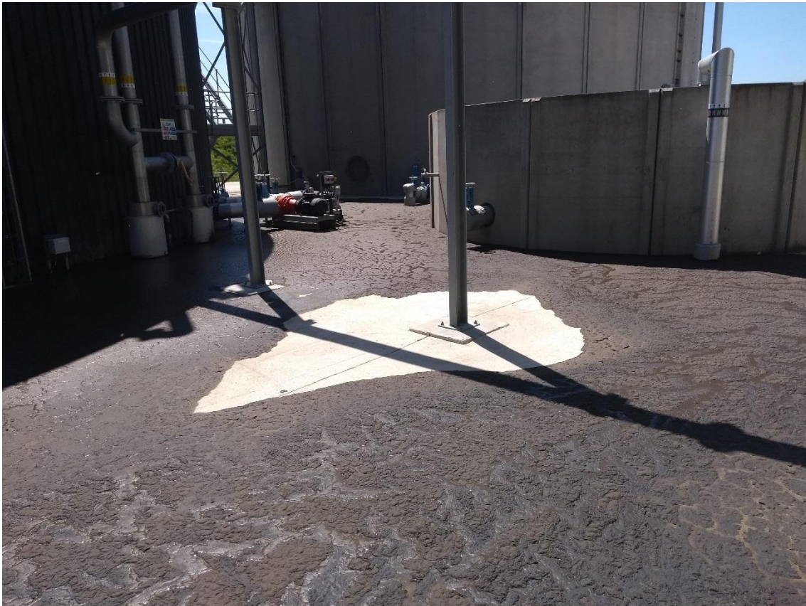
Figure 9: Residue from foam overflow incident.
