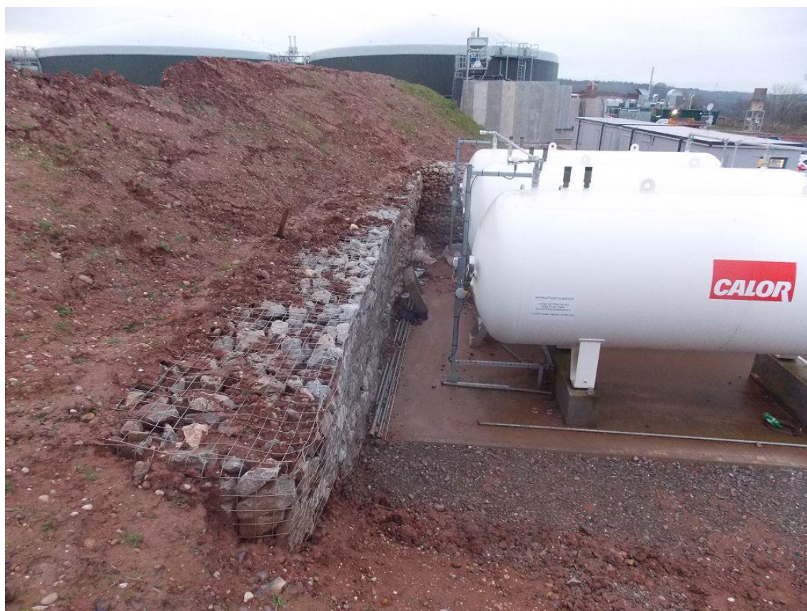
Figure 8: Bund collapse towards Propane Storage.
