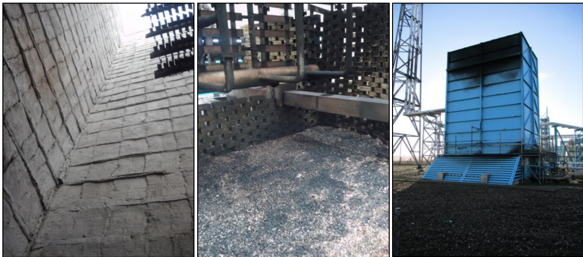
Figure 3: Inspection photographs of the ground flare following the event. Internal fire bricks (left), pipework and scorched gravel (pool fire residue) (middle) and soot deposits on external structure surface of the ground flare (right).
