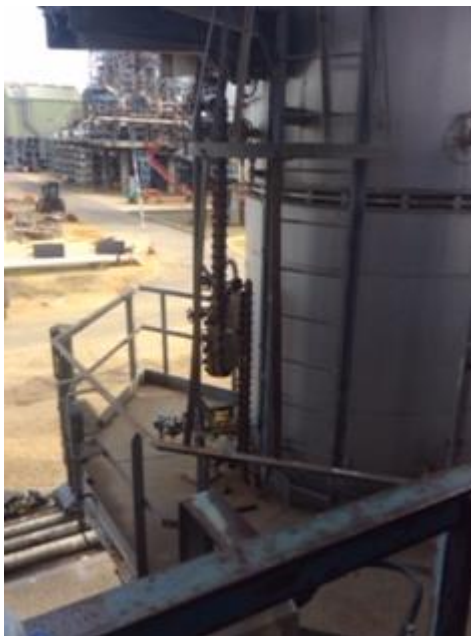
Figure 3: The P1 alarm tapping (painted yellow at the bottom of the ladder) is within the range of the BPCS level instrument
