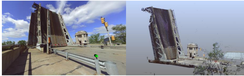
Figure 6: Photo (left) and Laser scan (right) of a damaged Bascule bridge.
