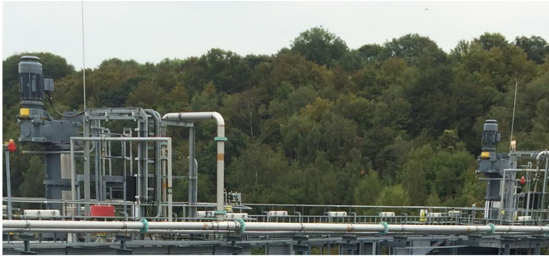
Image 4, air terminations on AD tank farm within ATEX zones.
