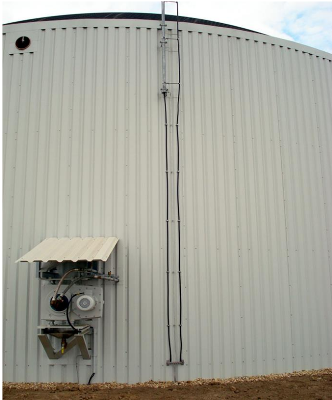
Image 9, LPS down conductor arrangement.
