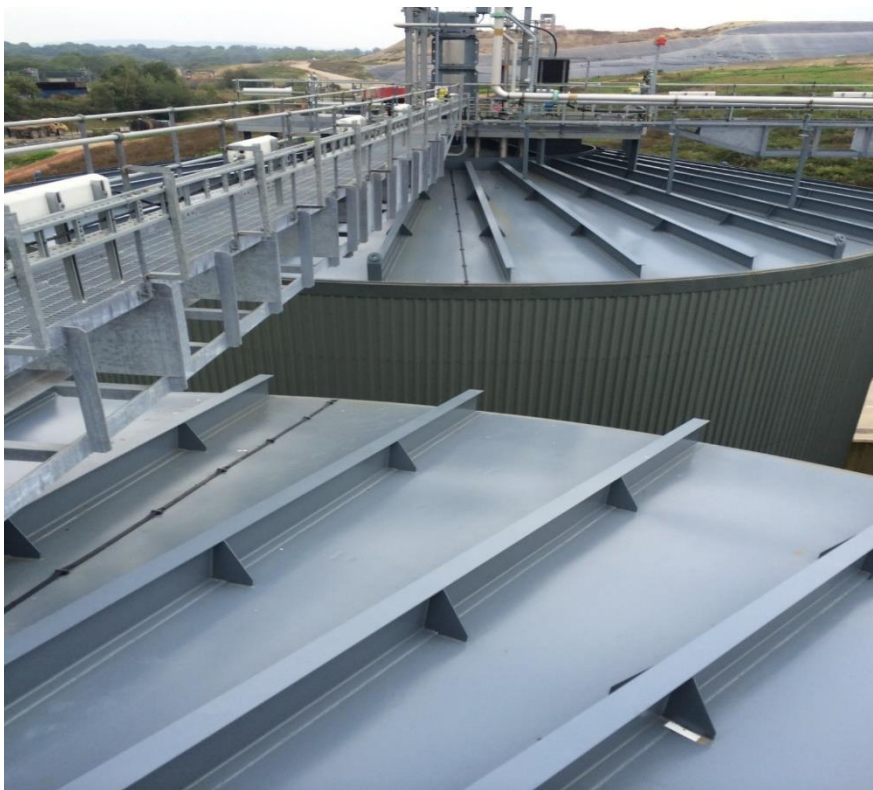
Image 3 Copper tape conductors on metallic AD tank farm.
