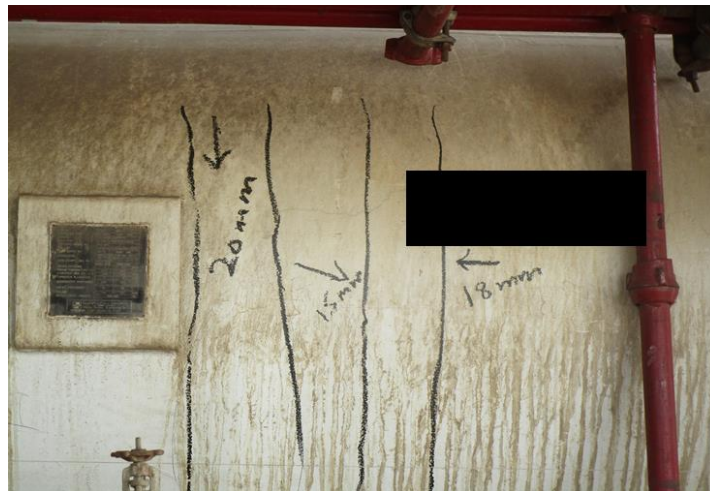
Figure 6. Evidence of bulged exchanger.
