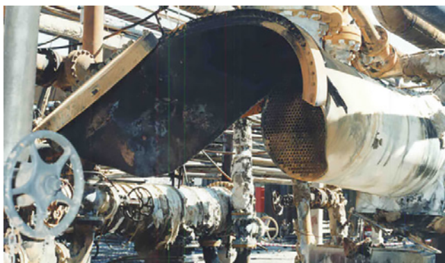
Figure 2 – ROD Reboiler GP905 after the accident
