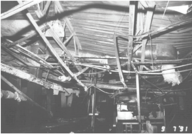
Figure 2 – Severe damage to steel girders and roof supports above the cooker vat
