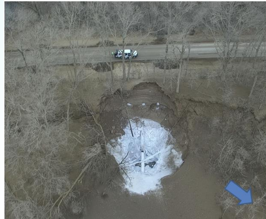
Reproduced from US Department of Transportation Pipeline and Hazardous Materials Safety Administration, Failure Investigation Report - Denbury Gulf Coast Pipelines, LLC 2022
