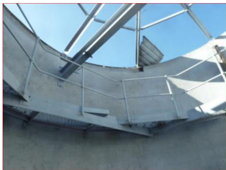
Figure 7: Roof blown off screen 1 silo tower
