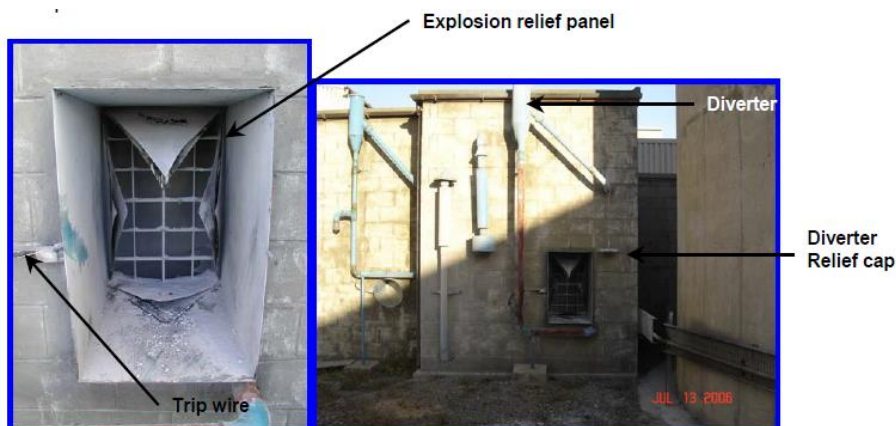
Figure 5: Vacuum filter no.2 explosion panel (LHS) and vent diverter (RHS)
