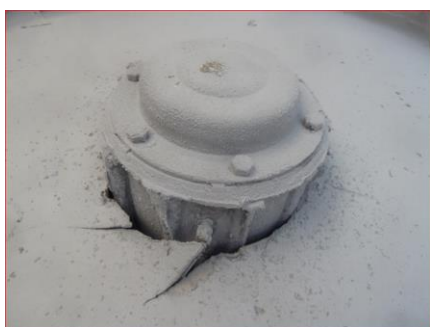
Figure 8: Bearing housing protruding through steel support area
