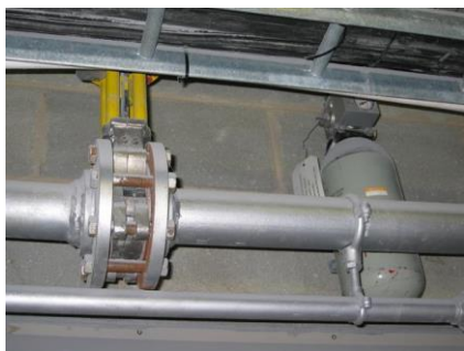
Figure 4: Rapid acting valve in vacuum suction line
