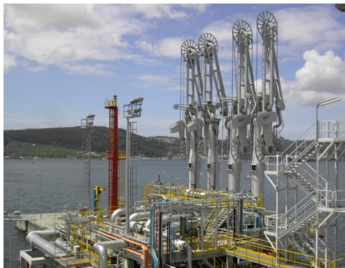
Figure 2. Marine transfer arms at Reganosa LNG Terminal, Spain.
