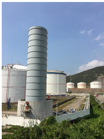
Figure 4. Enclosed ground flare- Shenzhen LNG Terminal, China.
