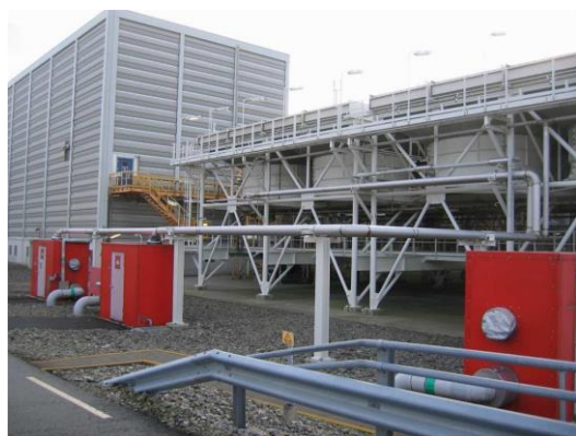
Figure 3 A gas compressor building where cladding provides explosion relief for internal explosion (hinged panels for projectile avoidance) and resistance to external explosions and 43dBA sound reduction
