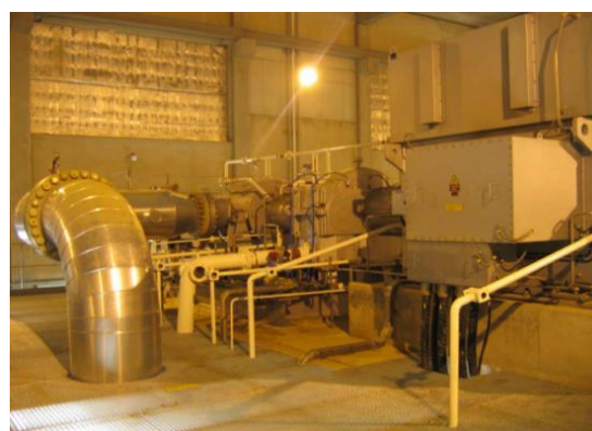
Figure 2 Explosion Relief panels viewed from inside, note foil- covered high density mineral fibre insulation for sound reduction and fire resistance.
