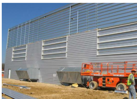
Figure 1 Stainless steel explosion relief panels installed on a gas compressor building in France
