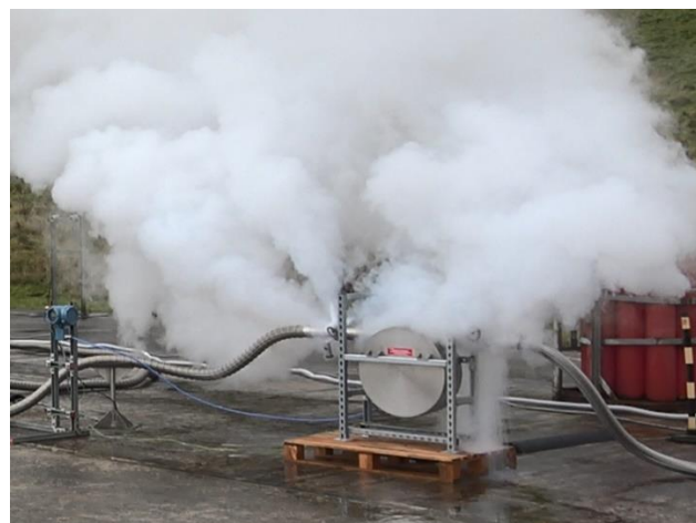
Figure 4: The leak on the upstream side of the flowmeter has progressed quickly to a large leak, it can be seen that it is impinging on the vacuum port of the hose. This occurred at 429 s into the experiment.
