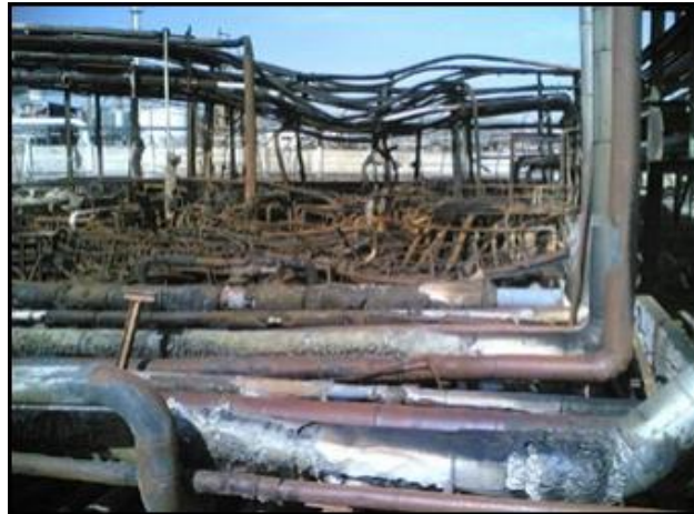
Fig. 2. The pipeline rack after the event
