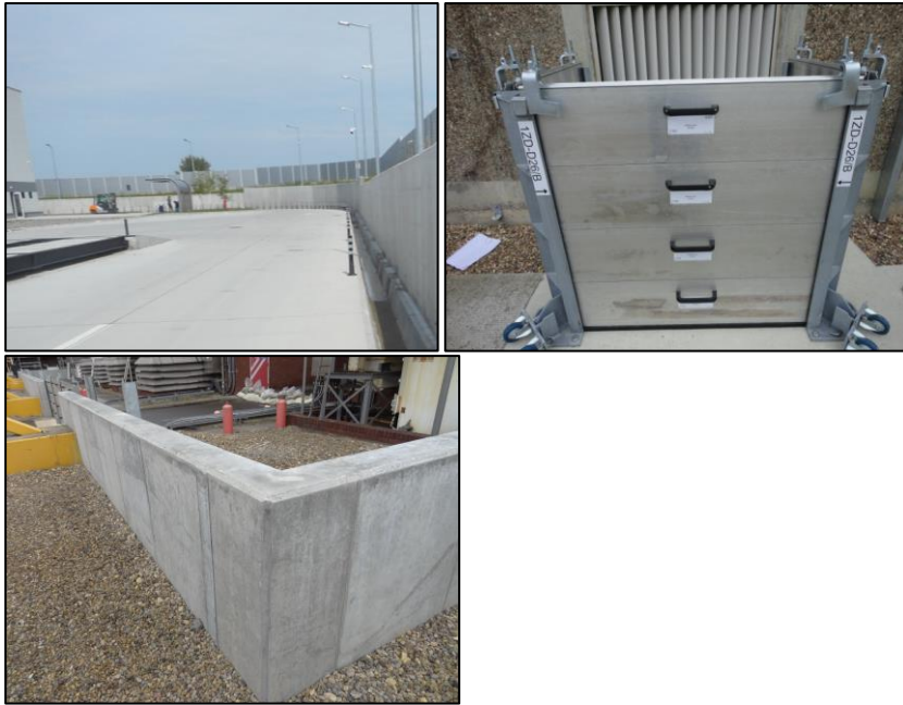
Figure 5. Building in Physical Layers of Protection – Primary Flood Walls, Secondary Building and Equipment Protection
