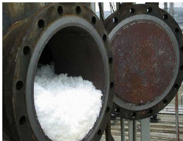
Figure 1 – Popcorn polymer in manhole (Credit: International Institute of Synthetic Rubber Producers Inc.)
