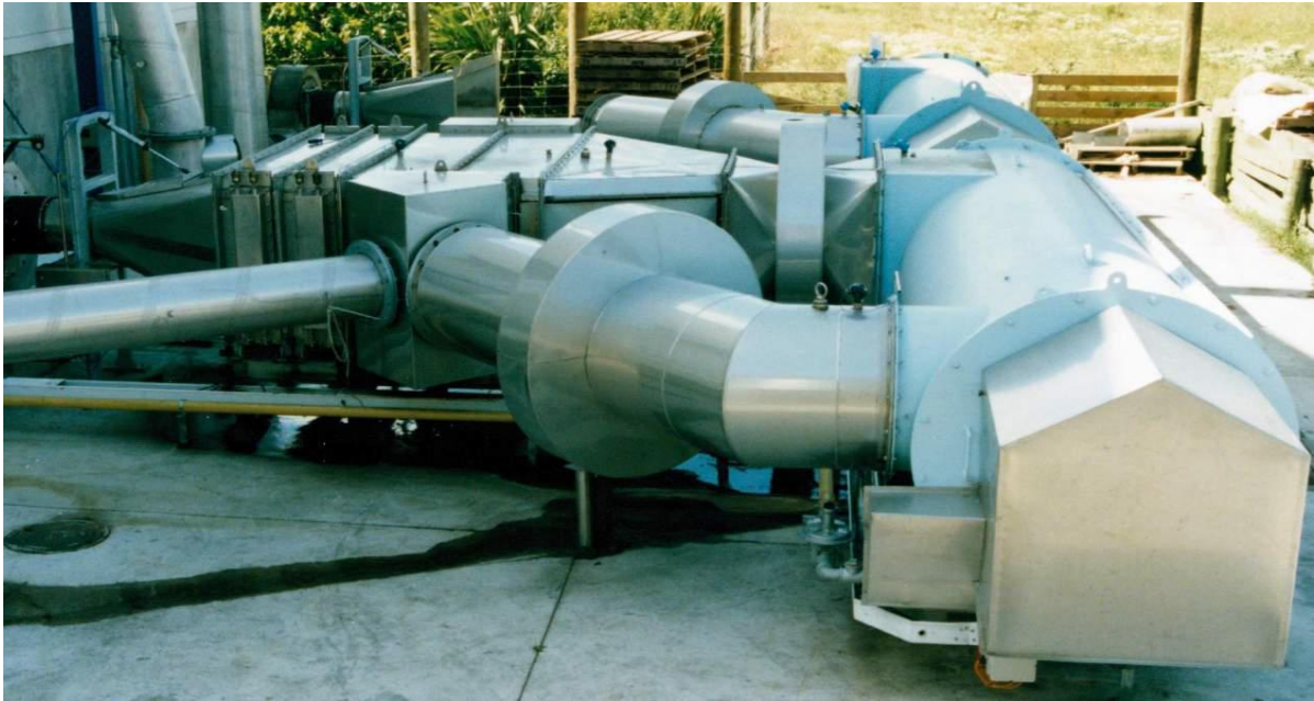
Recuperative After Burners PVLP Auckland 1994
