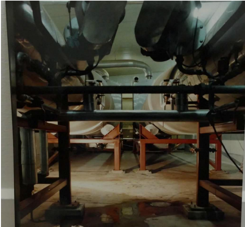
MLTR Plant 1987 - Dryers
