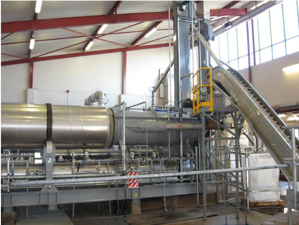
Demonstration Plant - First Stage Flo-Dryer
