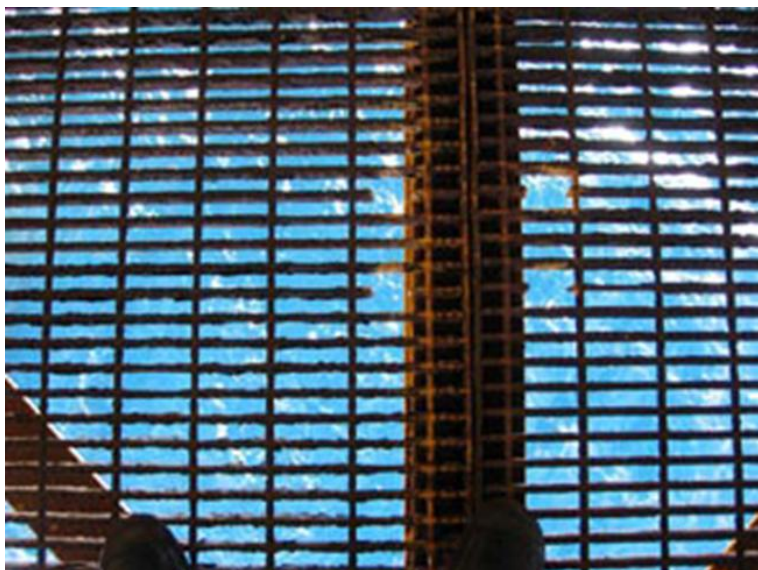
Figure 4: A close up view of the corroded gratings.
