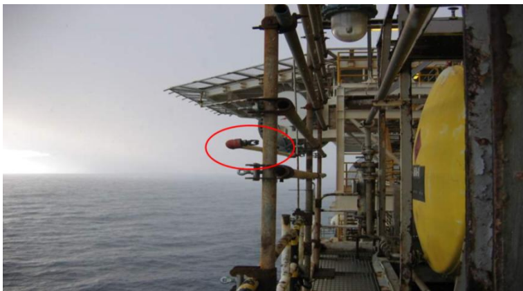
Figure 2: A deluge nozzle protecting a pressure vessel blocked by a scaffolding pole.
