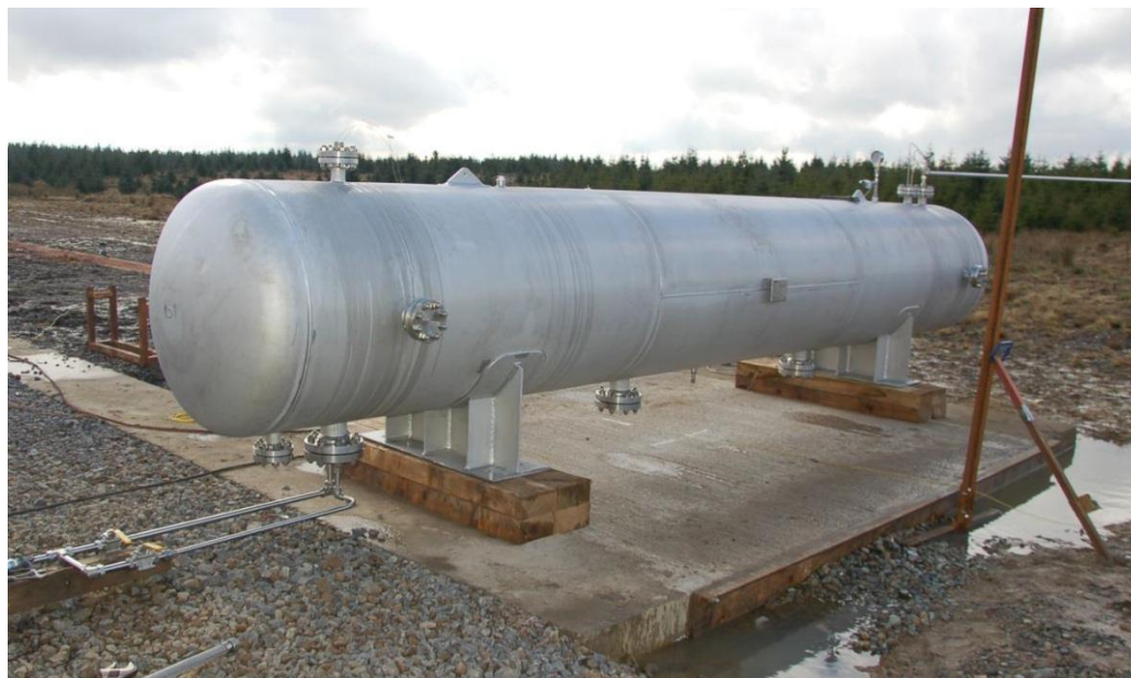
Figure 1: One of the three 5.055 m 3 pressurised vessels.
