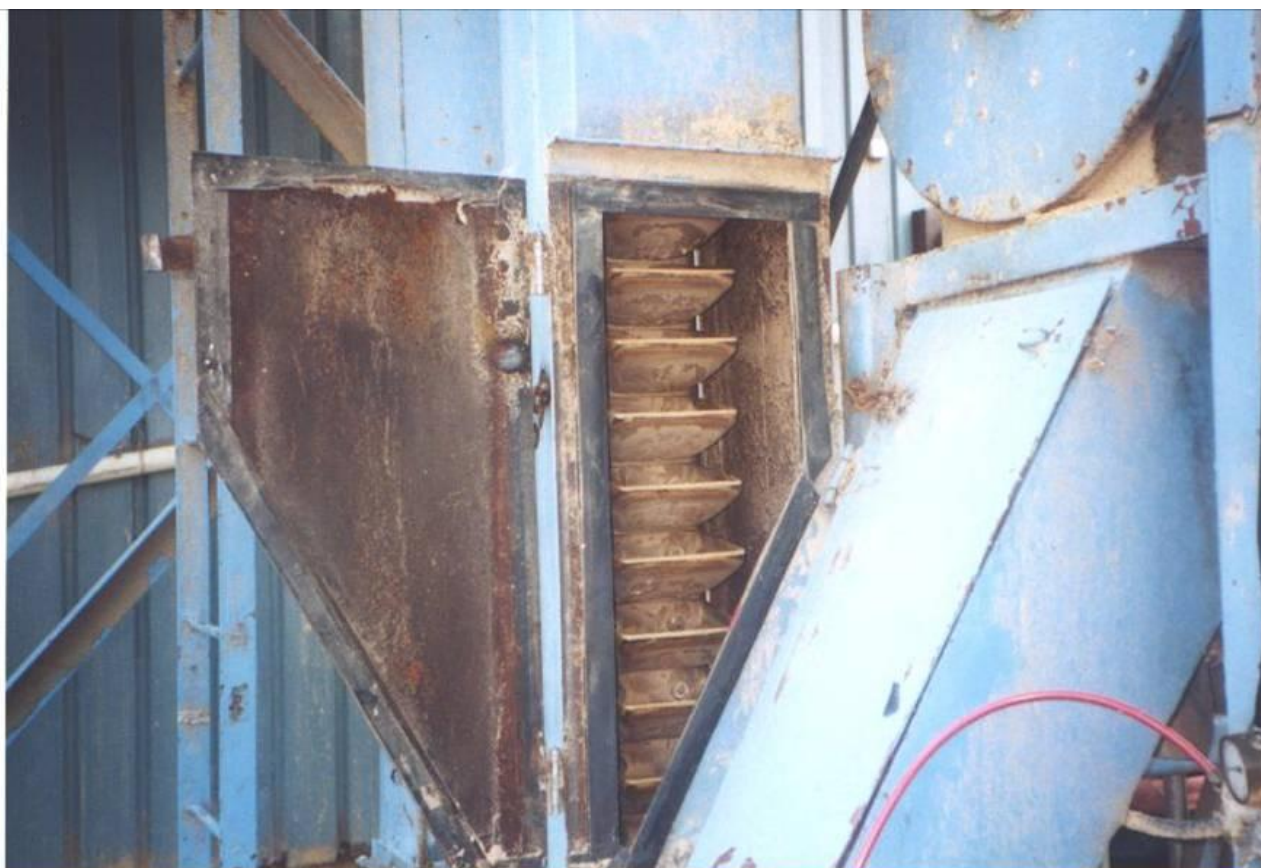
Figure 5 Uptake leg of bucket elevator with open panel showing individual buckets.
