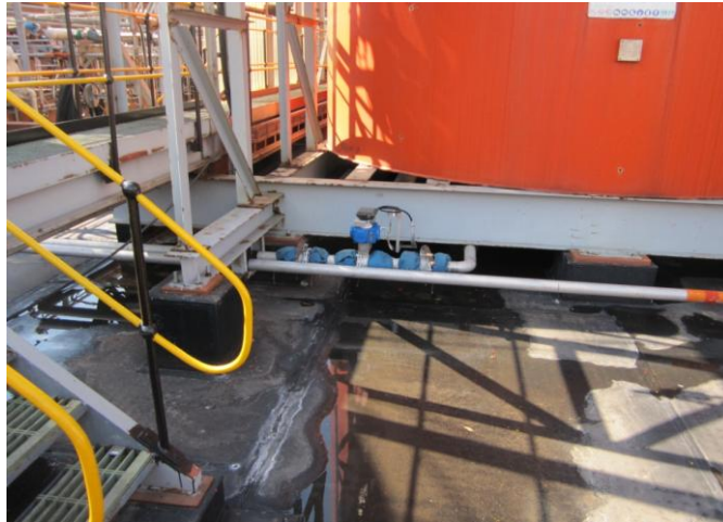
Figure 4: Equipment placed too low in acid tank sump
