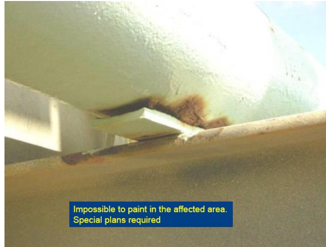
Figure 8: Erosion / corrosion issues are very difficult to see from the ‘outside’. Question the availability of thickness data for SCEs (Safety Critical Elements) like piping bends and T pieces.
