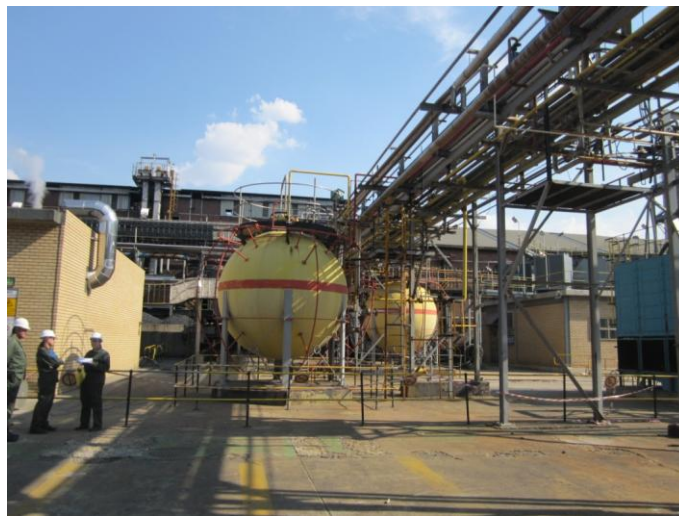
Figure 5: Hydrogen receivers too close to compressors and transformers – looks wrong!
