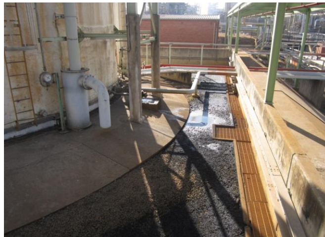
Figure 2: Unexplained leak from tank drain valve
