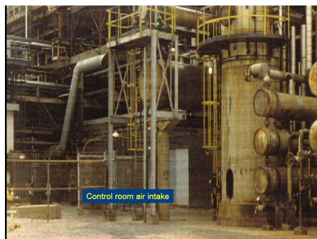
Figure 12: Air intakes may be fine in normal conditions. What can leak in the vicinity when an upset occurs or a LOC is experienced? The same thinking applies to venting at a “safe” distance.
